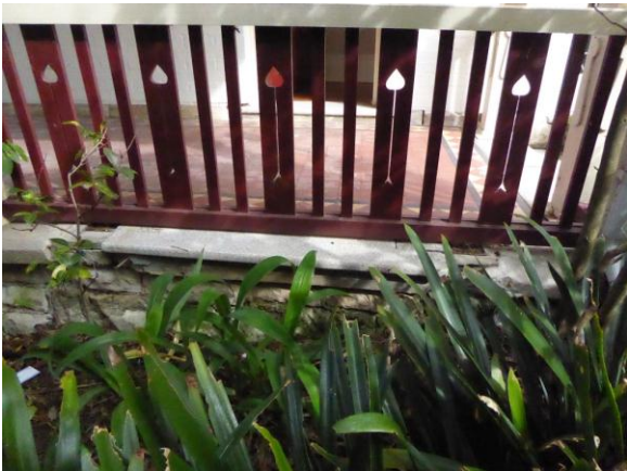
Figure 47: Later addition verandah balustrade showing evidence of location of original entry steps on east side of verandah
