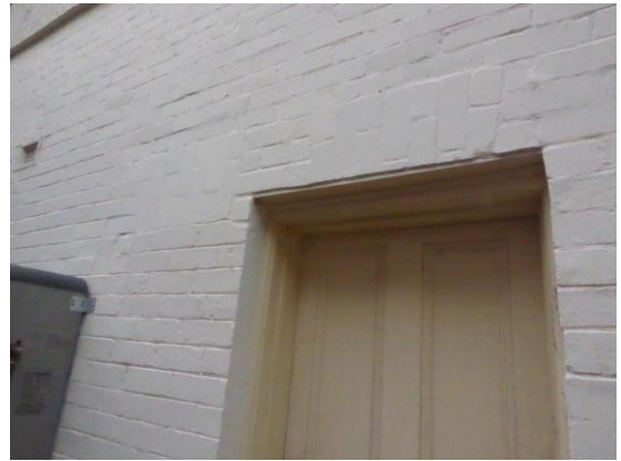
Figure 50: Evidence of location of former windows to west elevation with later addition door opening
