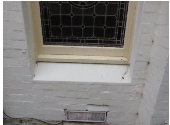
Figure 52: External view of leadlight window to dining room showing evidence that it is a later opening containing a relocated window.
