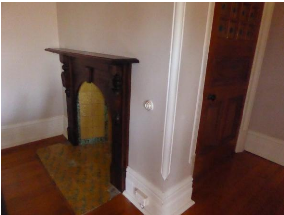
Figure 65: Later addition chimney piece with original (1890s) hearth tiles in sitting room
